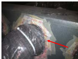
Improperly sealed duct connections
