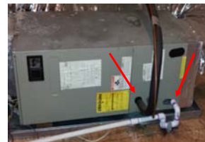
Unsealed penetrations in the cooling coil
