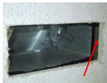
Gaps between Register boots and drywall
