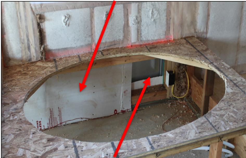
Metal access door needs to be insulated.
