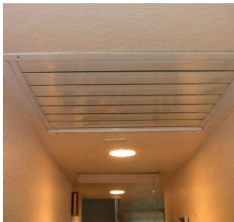
Figure 4-38: Whole-House Fan With Barometric Damper
