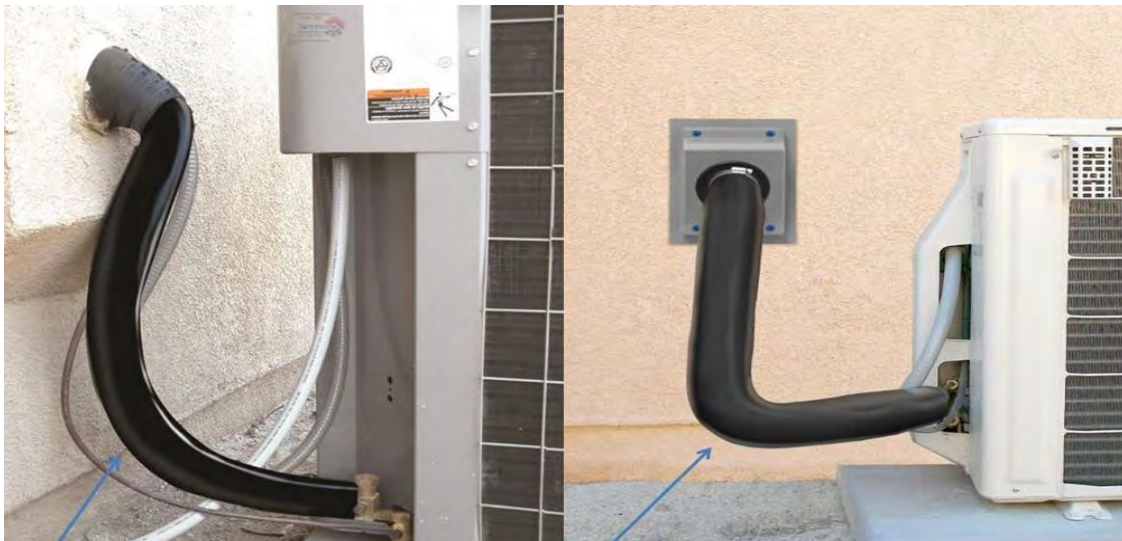
Figure 4-1: Refrigerant Line Insulation
