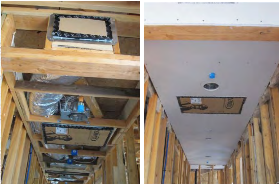
Figure 4-11: Ducts Routed Through a Dropped Ceiling
