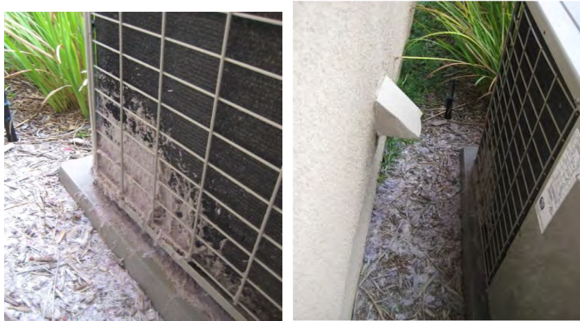
Figure 4-2: Noncompliant Condensing Unit Clearance From Dryer Vents
